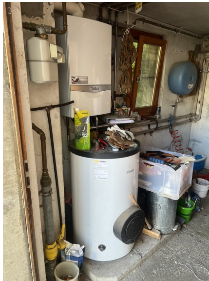
Existing Vaillant gas boiler (2018, 17 kW), official control 2024 — to be decommissioned and replaced by an air-water heat pump.
